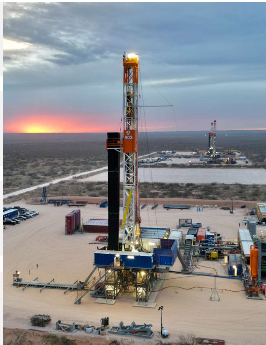
Guss well pad in Lea County, NM
