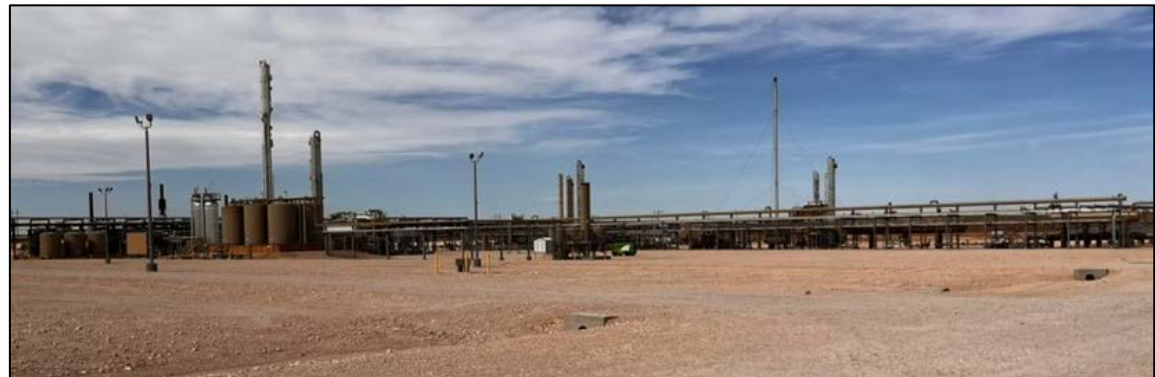
Pronto Midstream's Marlan Natural Gas Processing Plant
